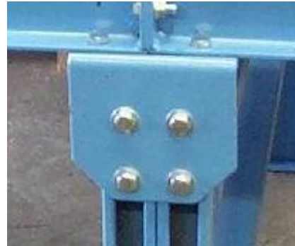
HD SUPPORT MOUNTED ON JOINT
